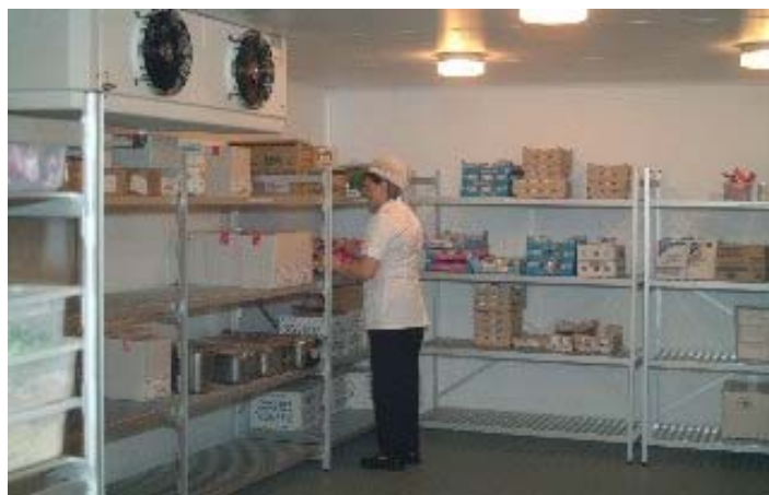
Foster coldroom with Duet Refrigeration system and Foster shelving
